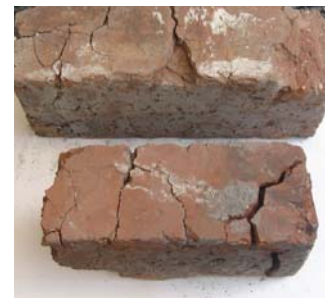
Photo 3- Exterior Cracked Bricks
