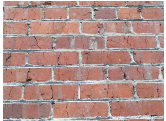
Photo 2- Cracking of bricks
